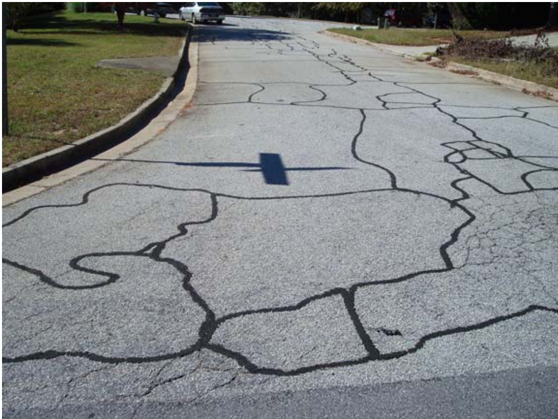
Picture of a crack sealed street
